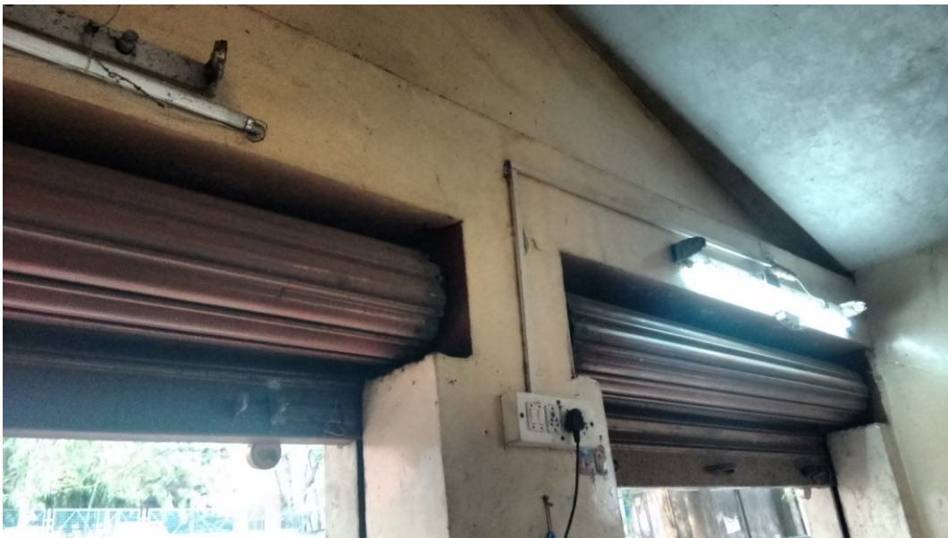
Figure 7. Improper lighting in the store
